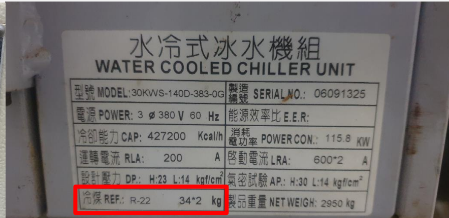
冰水機組銘牌拍照佐證
